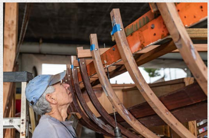
Volunteer Tim Stephens drills a hole to mount a new deck support.
